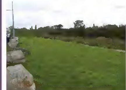
Figure 15.1 Filter strip at motorway service drainage to filter drain. Hapwood country (Brian Young)
